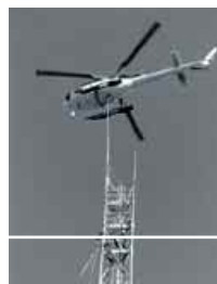
Installation of radio-communication antennas for Itinérís in southern France
